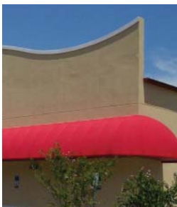
LEFT: Once erected, the panels took a minimal amount of infill to achieve the waved shapes. An acrylic stucco finish was then applied directly to the Koreteck panel surface.
